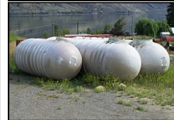
FIBREGLASS STORAGE TANKS 1-6000 GAL. 2-10,000 GAL.
