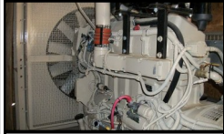
JOHN DEERE 425KW GENERATOR IN 40' TANDEM AXLE TRAILER
