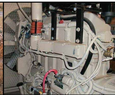
JOHN DEERE 425KW GENERATOR IN 40' TANDEM AXLE TRAILER
